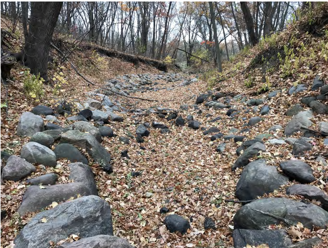
Figure 18. Bank stabilization and grade control in the middle of the Kici Yapi reach
