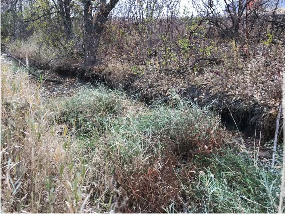
Figure 3. Bank erosion downstream of Fountain Hills Road
