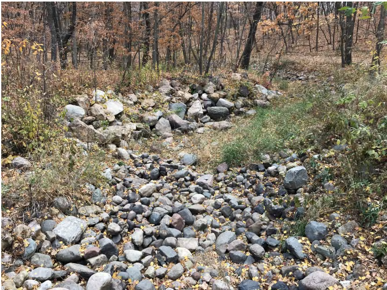
Figure 16. Rock bank stabilization at the upstream end of the Kici Yapi reach
