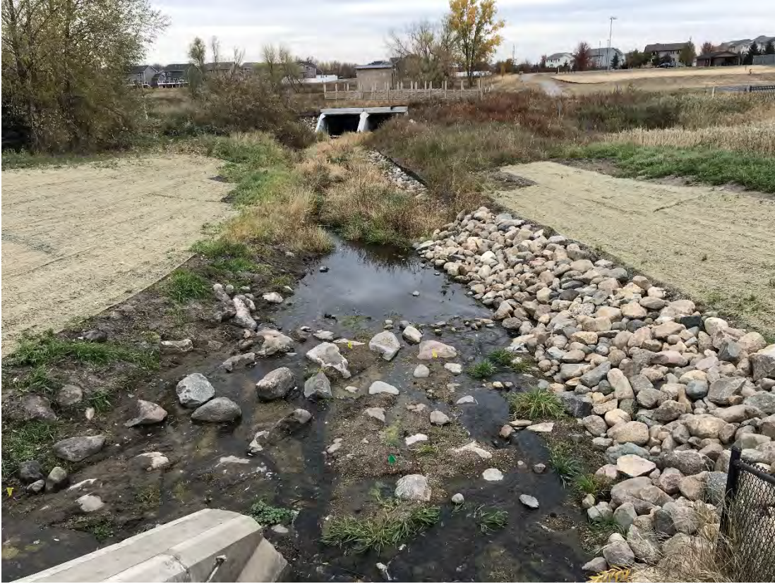
Figure 36. New box culvert installed at the upstream end of the new channel alignment in Segment 5B
