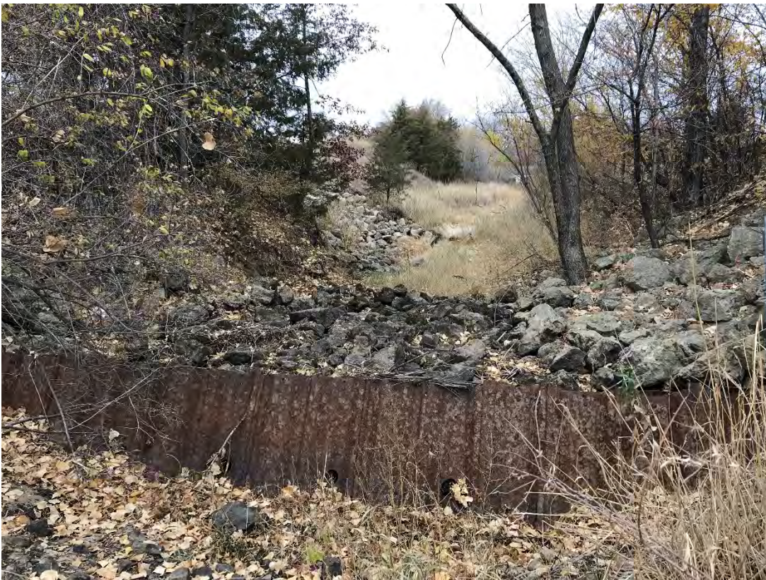
Figure 48. Corroded sheet pile weir in Segment 7A
