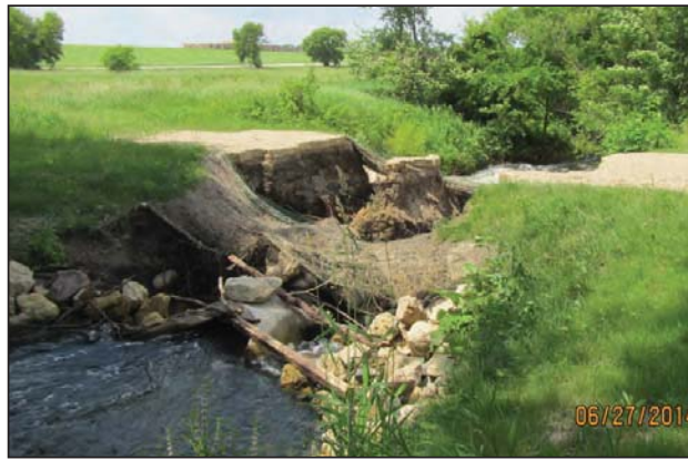
Damaged culverts along the Prior Lake Outlet Channel will be among the repairs made next year using state and federal disaster relief funds.
